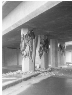
Figure 2.3. Failure of columns of the Route 5/210 interchange during the 1971 San Fernando earthquake.
