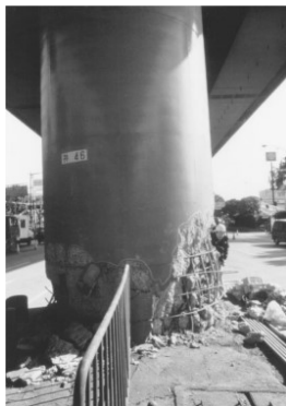
Figure 2.4. Hanshin Expressway, Pier 46, damage in the 1995 Hyogo-Ken Nanbu earthquake.
