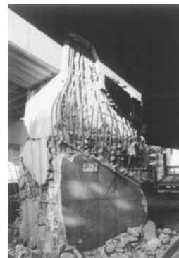
Figure 2.5. Failure of column with longitudinal reinforcement cut-offs near midheight in the 1995 Hyogo-Ken Nanbu earthquake.
