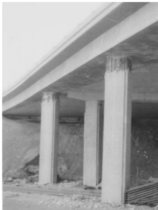
Figure 2.2. San Fernando Road Overhead damage in the 1971 San Fernando earthquake.
