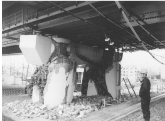
Figure 2.6. Failure of a two-column bent in the 1995 Hyogo-Ken Nanbu earthquake.
