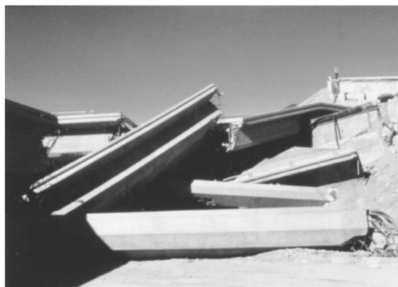
Figure 2.7. Failure at the base of a column supported on a single cast-in-place pile in the 1971 San Fernando earthquake.
