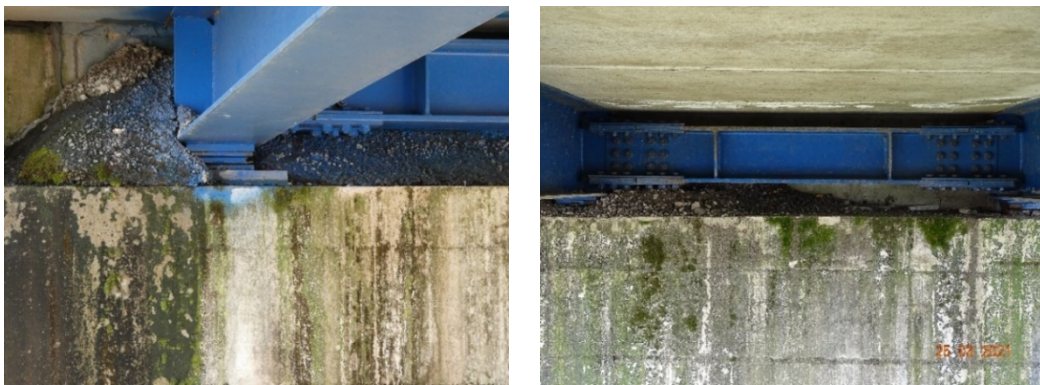
Figure 35 - Presence of debris
