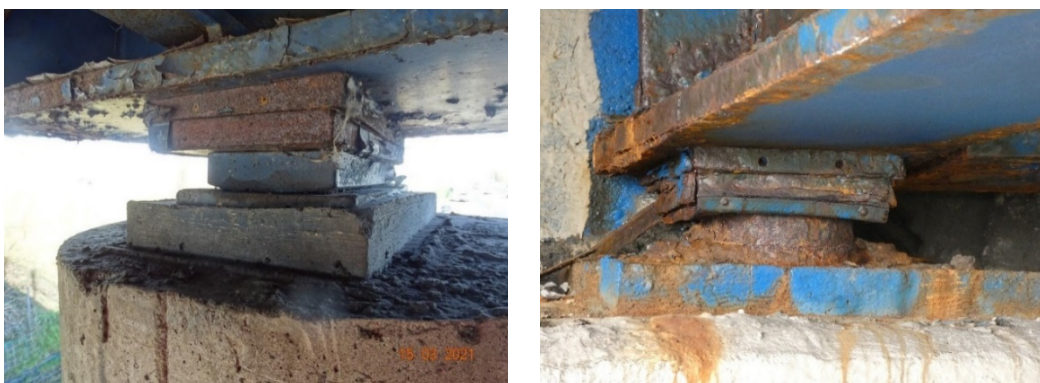
Figure 32 - Bearing device rusting
