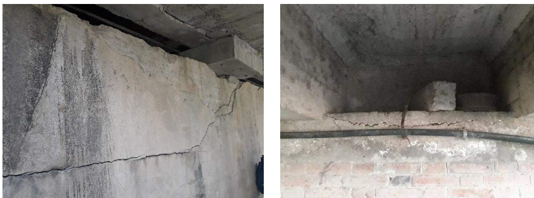
Figure 40 - Characteristic cracks at the support location (Adopted from Annex C of the Italian guidelines)
