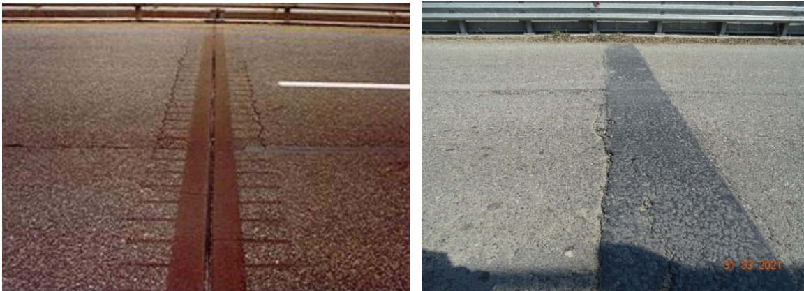
Figure 42 – Left: damaged screeds; Right: gap plug deformation (Adopted from Annex C of the Italian guidelines)
