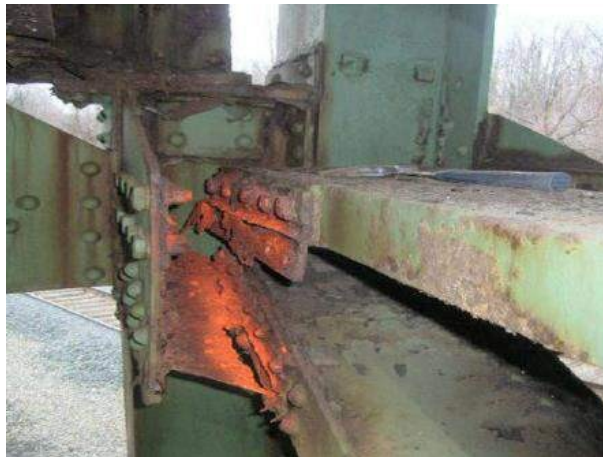
Figure 15 - Joint damage (Adopted from Annex C of the Italian guidelines)
