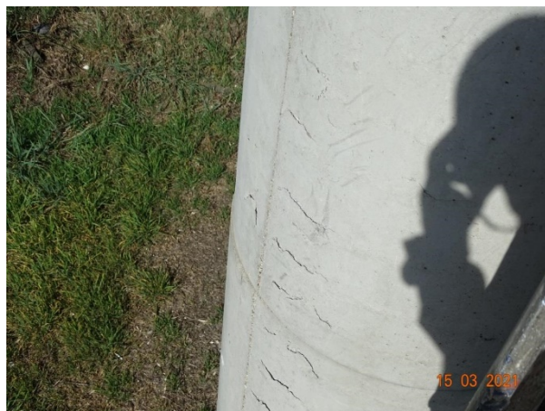
Figure 28 - Cracks at the stirrup position
