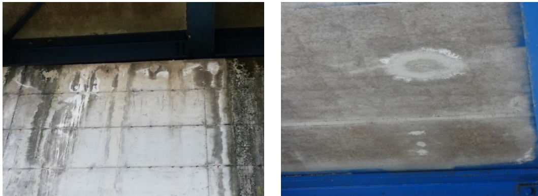
Figure 18 - Passive moisture stains
