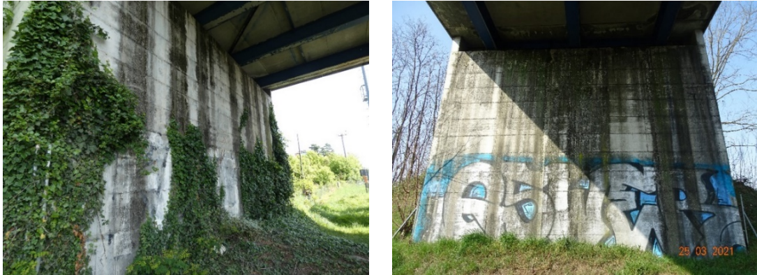
Figure 19 - Active moisture stains
