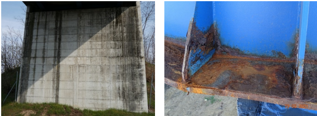
Figure 38 – Left: Drainage marks; Right: Water stagnation.
