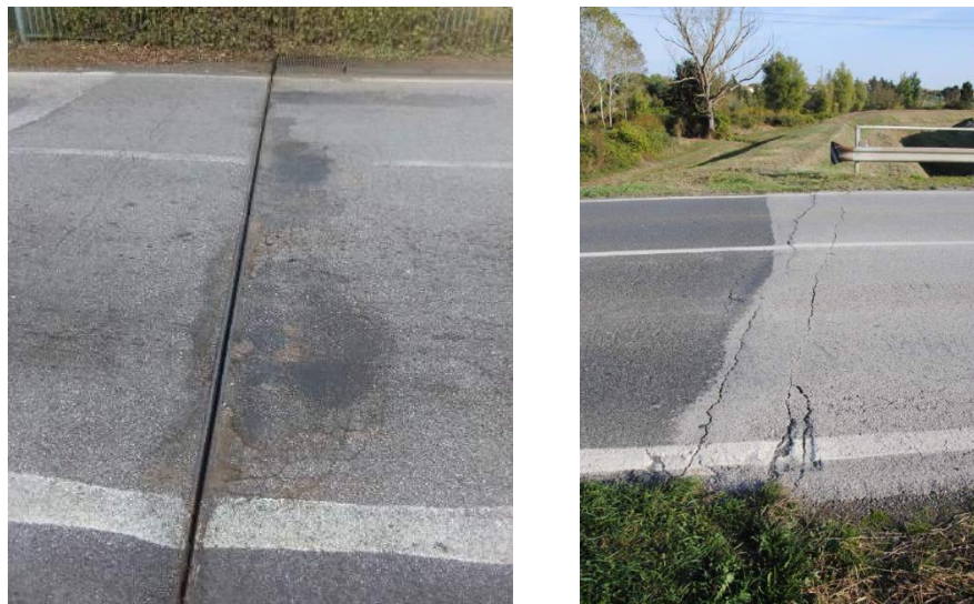
Figure 41 – Left: Pavement-expansion joint gap; Right: Gap plug detachment (Adopted from Annex C of the Italian guidelines)
