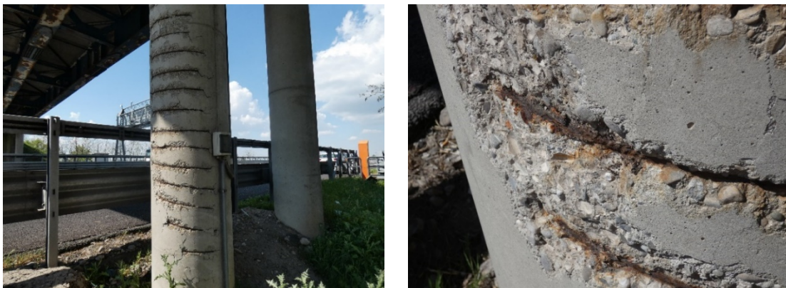
Figure 29 - Rusted and/or corroded stirrups
