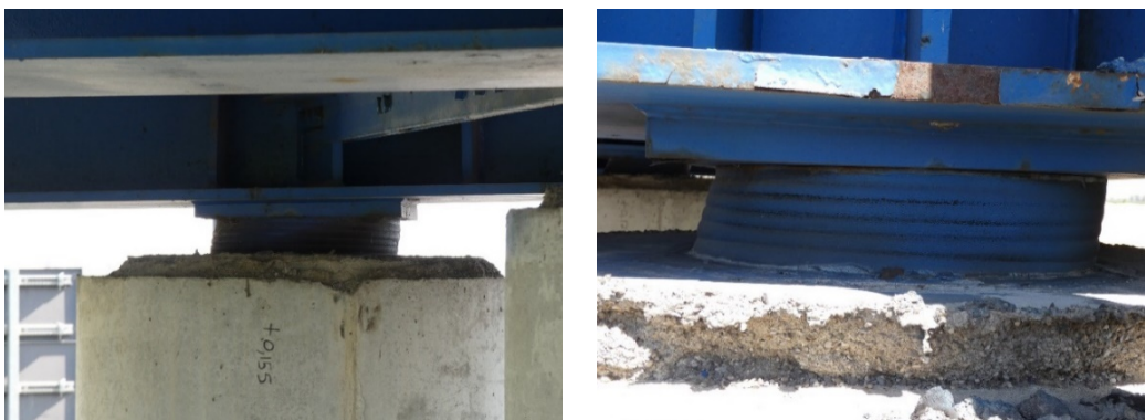
Figure 37 - Excessive lateral deformation of neoprene
