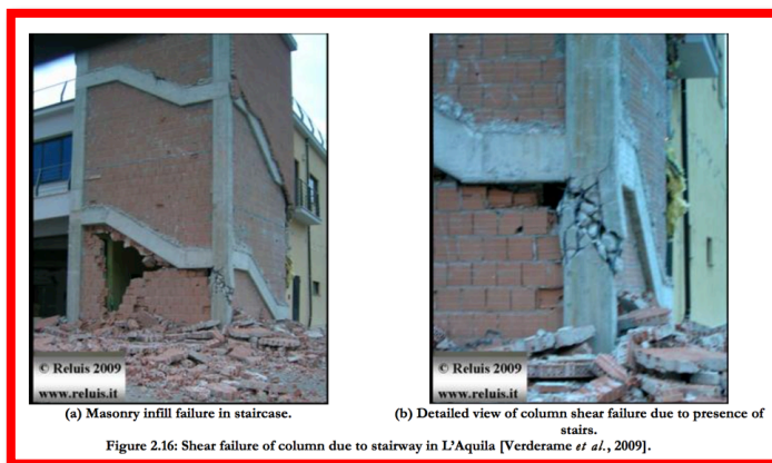
Figure 2.16: Shear failure of column due to stairway in L'Aquila [Verderame et al. , 2009].
