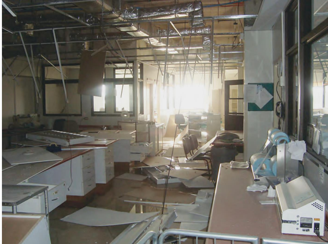
Photo by Bill Holmes, Rutherford & Chekene (FEMA E-74, Fig. 6.3.4.1-3). 2010 M8.8 Chile earthquake
