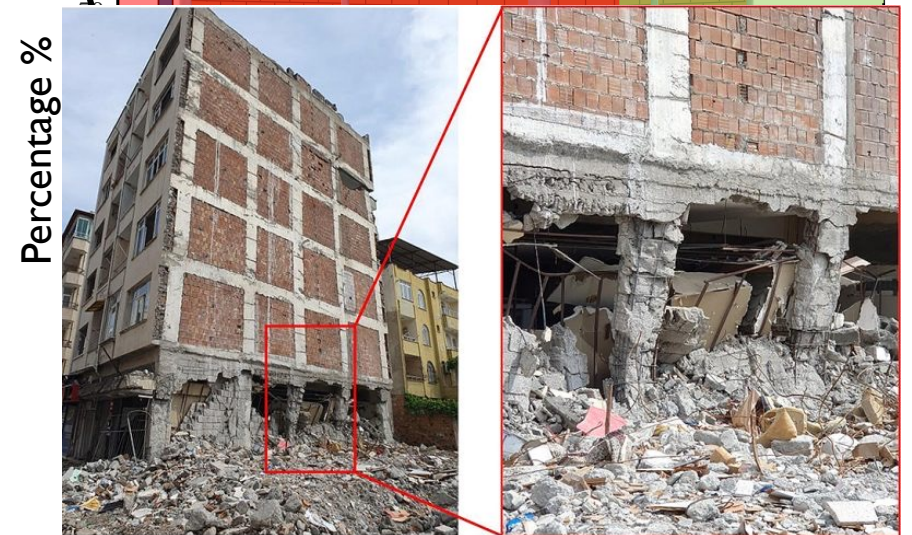
Joint Reconnaissance EUCENTRE-ReLUI5, Turkey-Syria Earthquake 2023 - Final report
